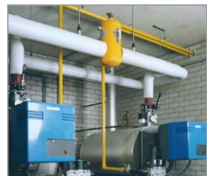
Deaerator in a utility plant
